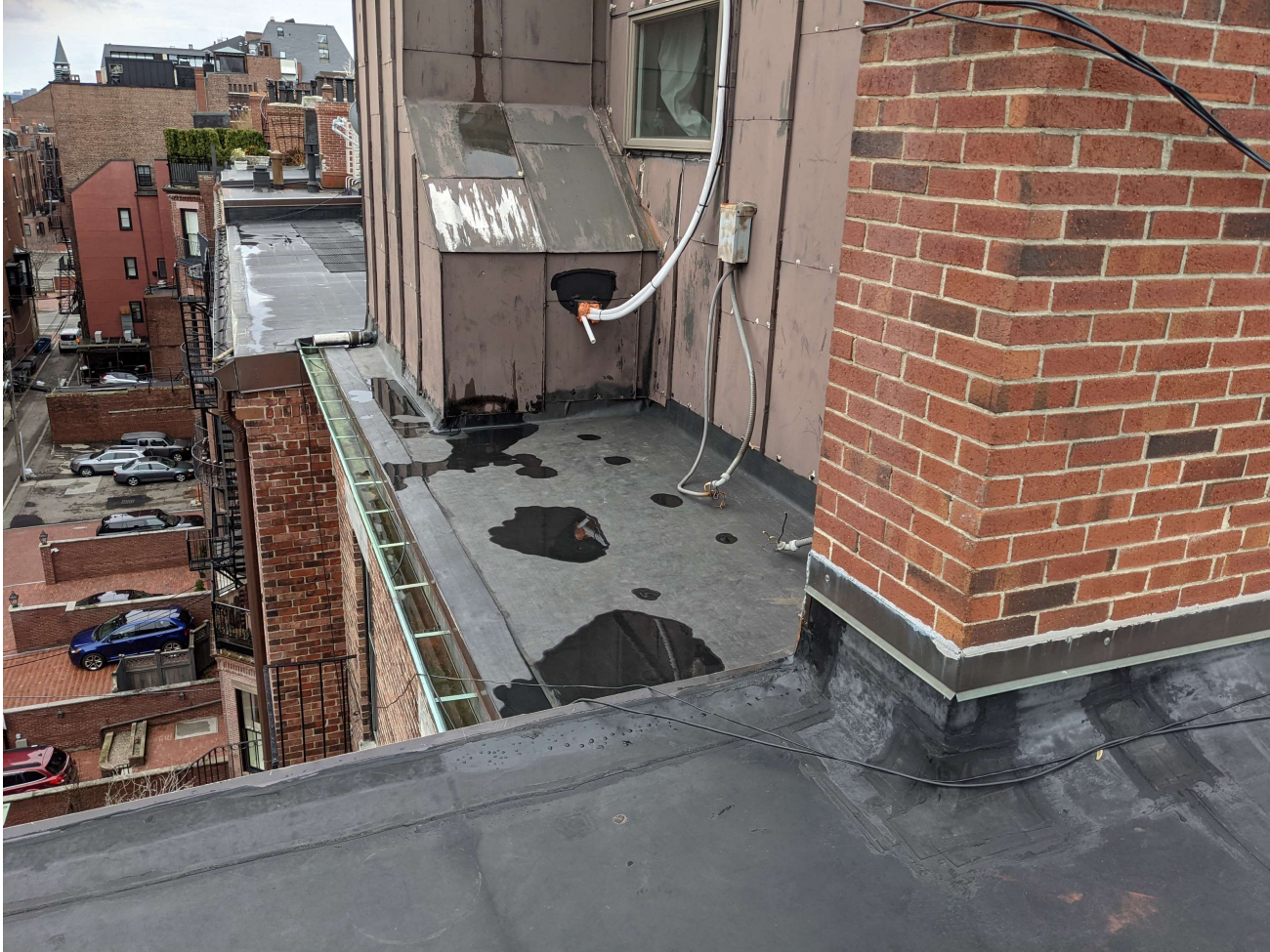
Common Mechanical Equipment Area For Building
