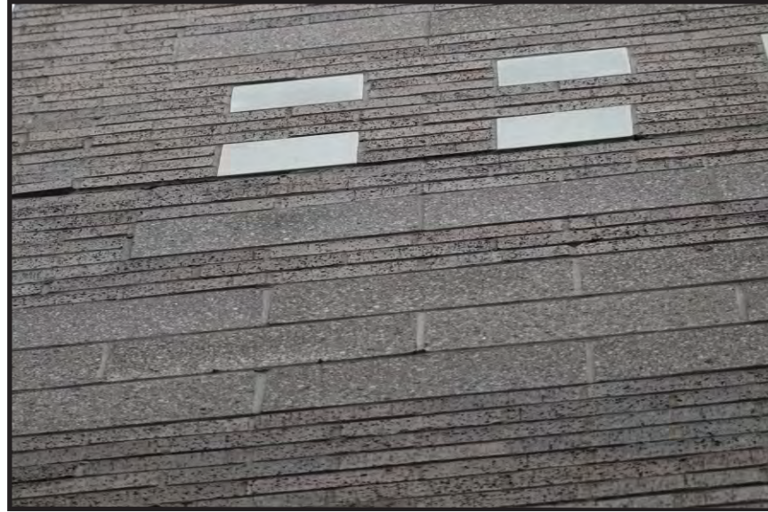
FAILED SEALANT JOINT, OPENING THE BUILDING FACADE FOR WATER AND FREEZE THAW DAMAGE.
