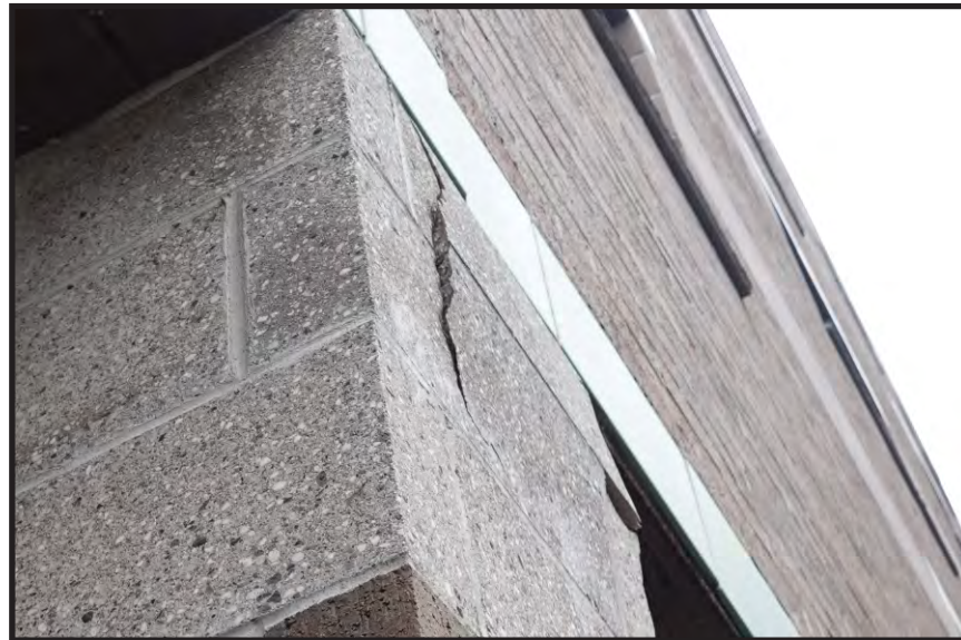
STEEL LINTEL IS RUST JACKING THE MASONRY, OPENING THE BUILDING FACADE FOR WATER AND FREEZE THAW DAMAGE.
