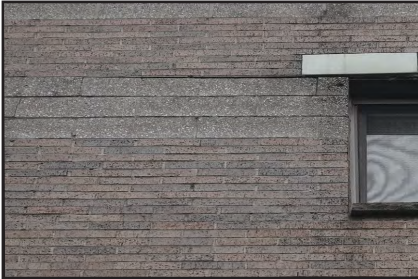
STEEL LINTEL AT WINDOW IS RUST JACKING THE MASONRY, OPENING THE BUILDING FACADE FOR WATER AND FREEZE THAW DAMAGE.
