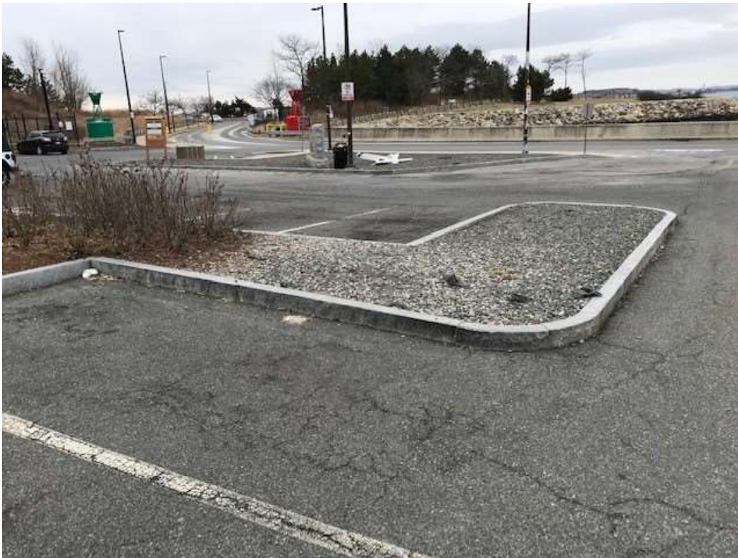
Photograph 3. View of one of the stone areas to be converted to parking, facing south.
