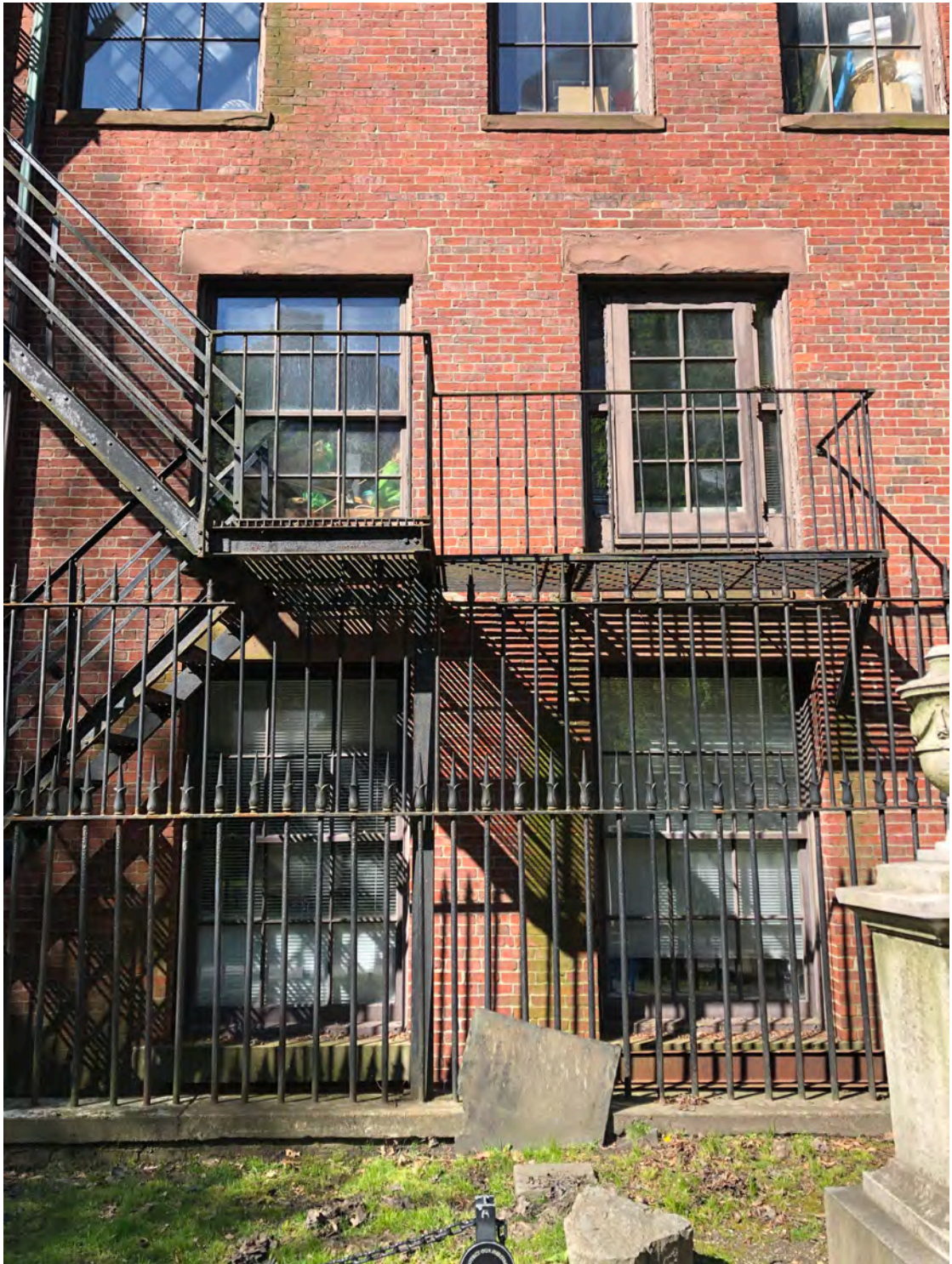
REAR FACADE AT SECOND FLOOR EXIT DOOR TO FIRE ESCAPE; REMOVE EXTENDED FIRE ESCAPE LANDING; REMOVE EXIT DOOR & RESTORE MISSING WINDOW
