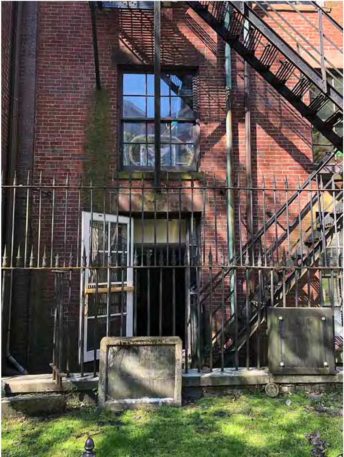
REAR FACADE AT FIRST FLOOR EXIT DOOR TO FIRE ESCAPE; REMOVE FIRST FLOOR EXIT DOOR & RESTORE MISSING WINDOW
