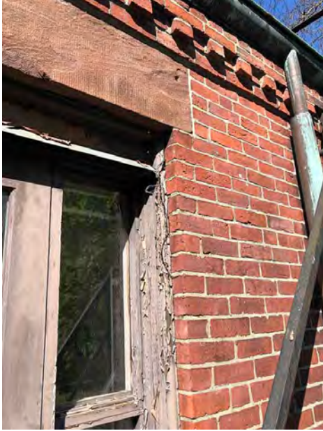
SCABBLE OFF FRIABLE STONE LINTEL AND PROVIDE MATCHING REPAIR MORTAR TO RESTORE SURFACE
