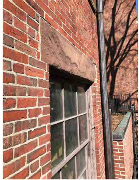
SCABBLE OFF FRIABLE STONE AND APPLY MATCHING REPAIR MORTAR TO RESTORE SURFACE OF LINTEL
