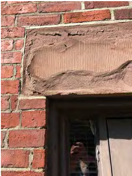
SAWCUT DEEPLY ERODED PORTIONS OF STONE & FIT WITH BONDED DUTCHMAN; SCABBLE OFF FRIABLE SURFACE & RESTORE WITH MORTAR TO MATCH
