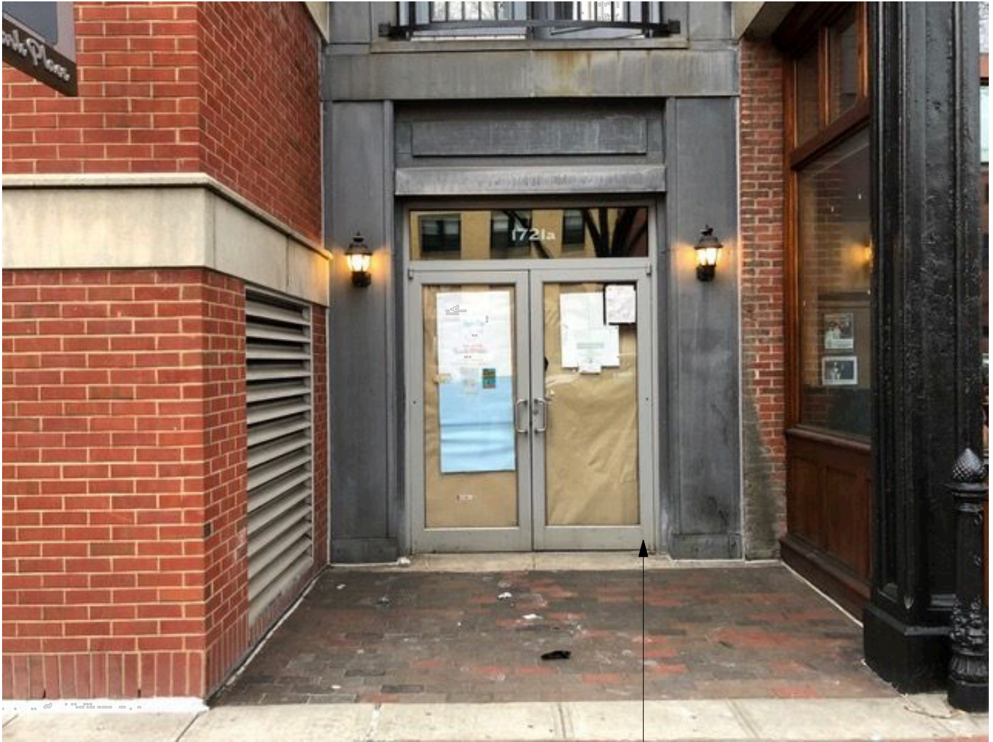
EXISTING FRONT DOOR TO BE REPLACED
