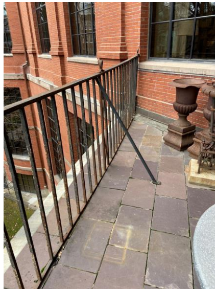
Photo 3: Non-original railing at second-floor balcony does not comply with current architectural or structural code.
