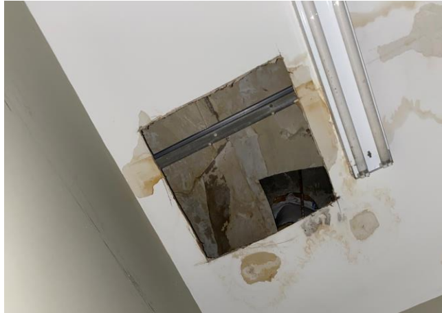
Photo 2: Interior water damage below second-floor balcony.
