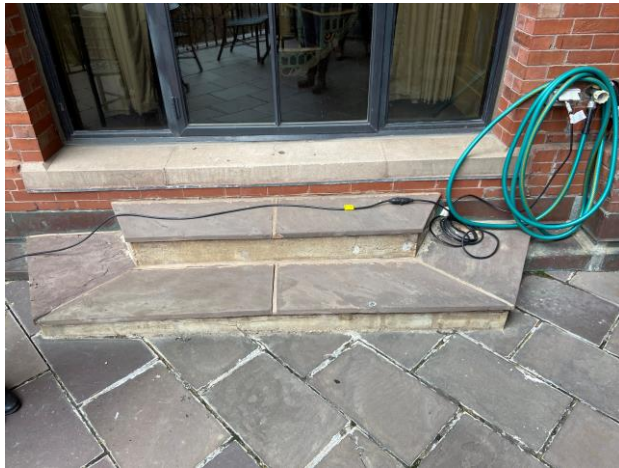
Photo 4: Slippery and loose pavers at edge and stairs pose potential tripping hazards.
