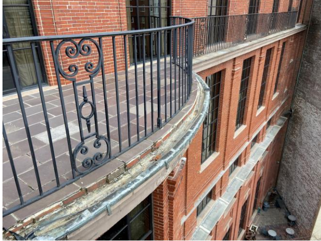
Photo 5: Slippery and loose pavers pose potential tripping hazards and non-original railing at fifth-floor does not comply with current architectural or structural code.
