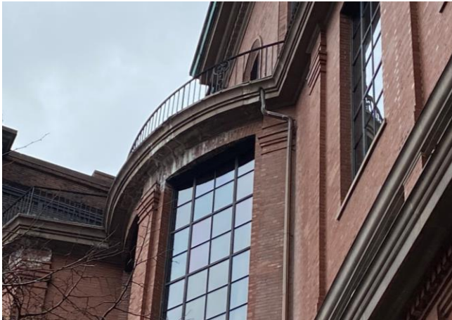
Photo 7: Mortar-set pavers and leaking gutter are contributing to masonry staining and deterioration below the fifth-floor balcony.
