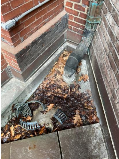
Photo 1: Clogged internal drain at second-floor balcony
