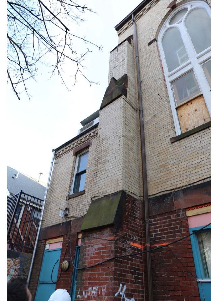
Buttress with old patches and repairs (Spring 2019)
