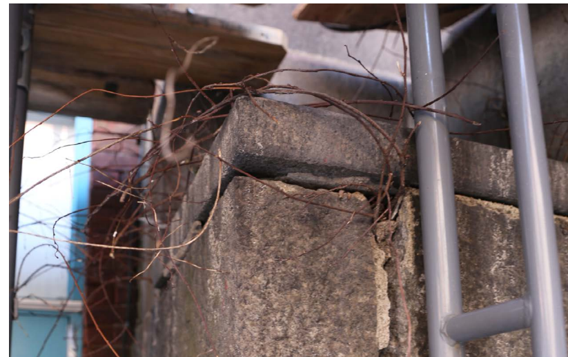
Stone displacement in granite base (Spring 2019)
