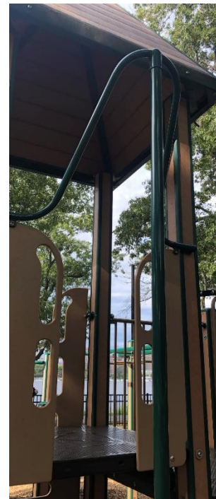
Non-compliant Fire pole
