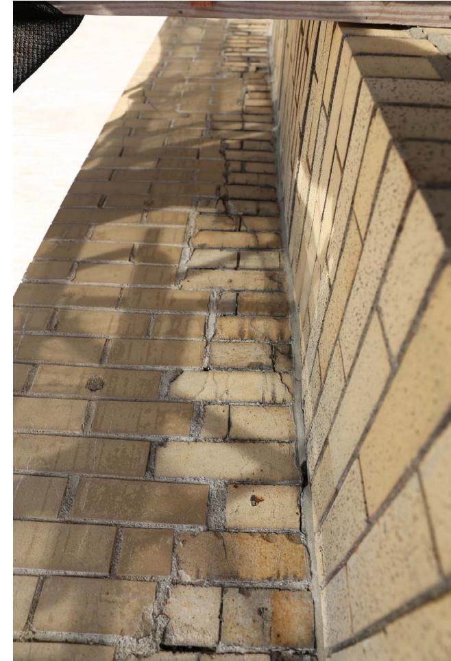
Cracks, tests and old repairs (Spring 2019)
