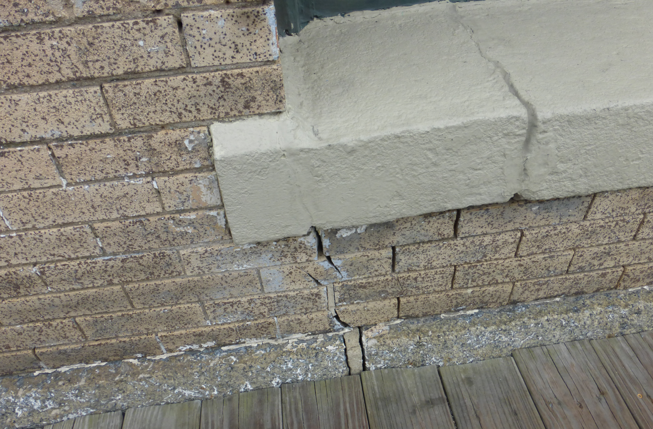
9. VIEW AT CRACK FACADE AT HARBORWALK
