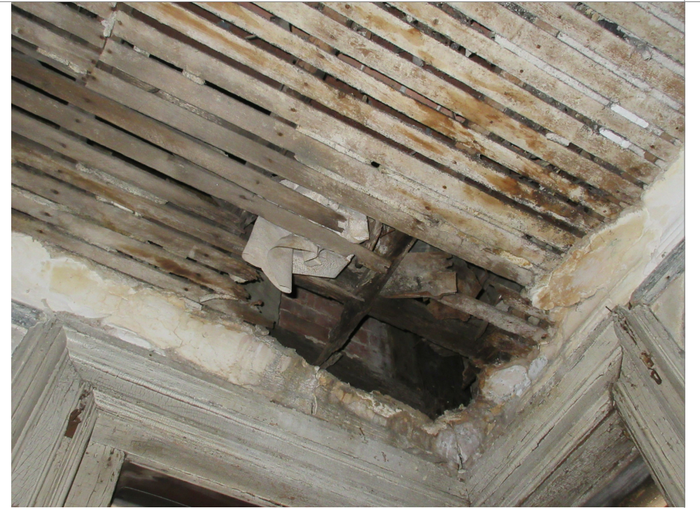
WATER DAMAGE AT CEILING
