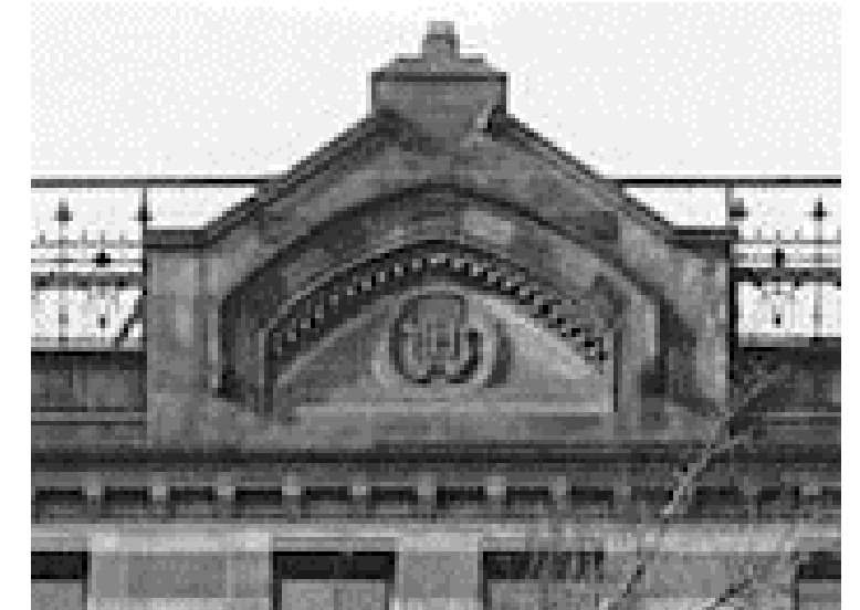
PHOTO 7: ORIGINAL SANDSTONE GABLE DETAIL TO BE REPLICATED WHERE DETAILS ARE NOW MISSING
