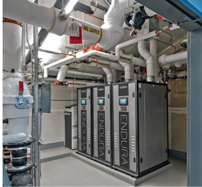
▶ Three Endura boilers are integrated directly into a primary-only variable flow installation to provide building heat.
