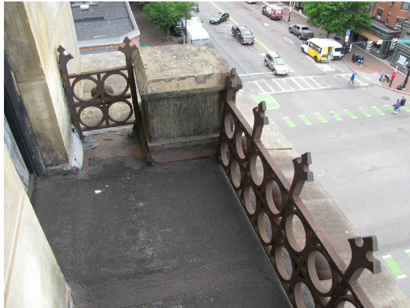
PHOTO 1: EXISTING BALCONY CAST IRON RAIL ON THE SOUTH ELEVATION. REPLICATE EXISTING BALCONY RAIL WHERE MISSING ON SOUTH AND EAST ELEVATIONS.
