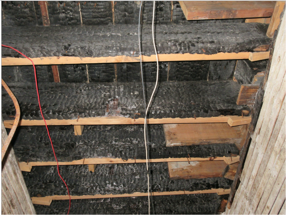
FIRE DAMAGE AT FLOOR FRAMING
