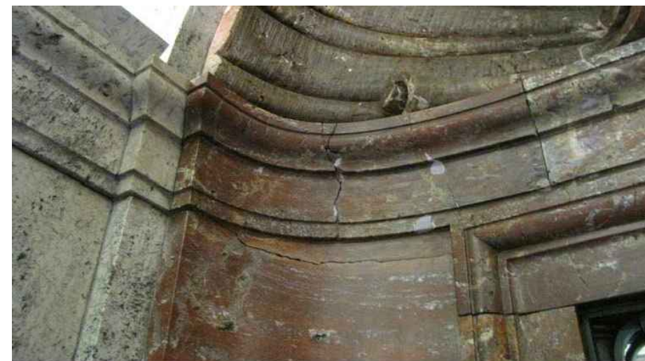
PHOTO 3: CRACK IN STONE WALL
