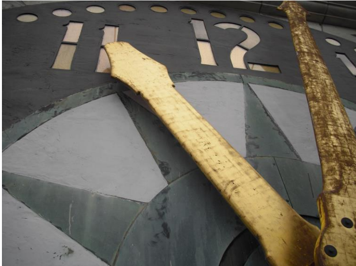
Deteriorated gold leaf finish
