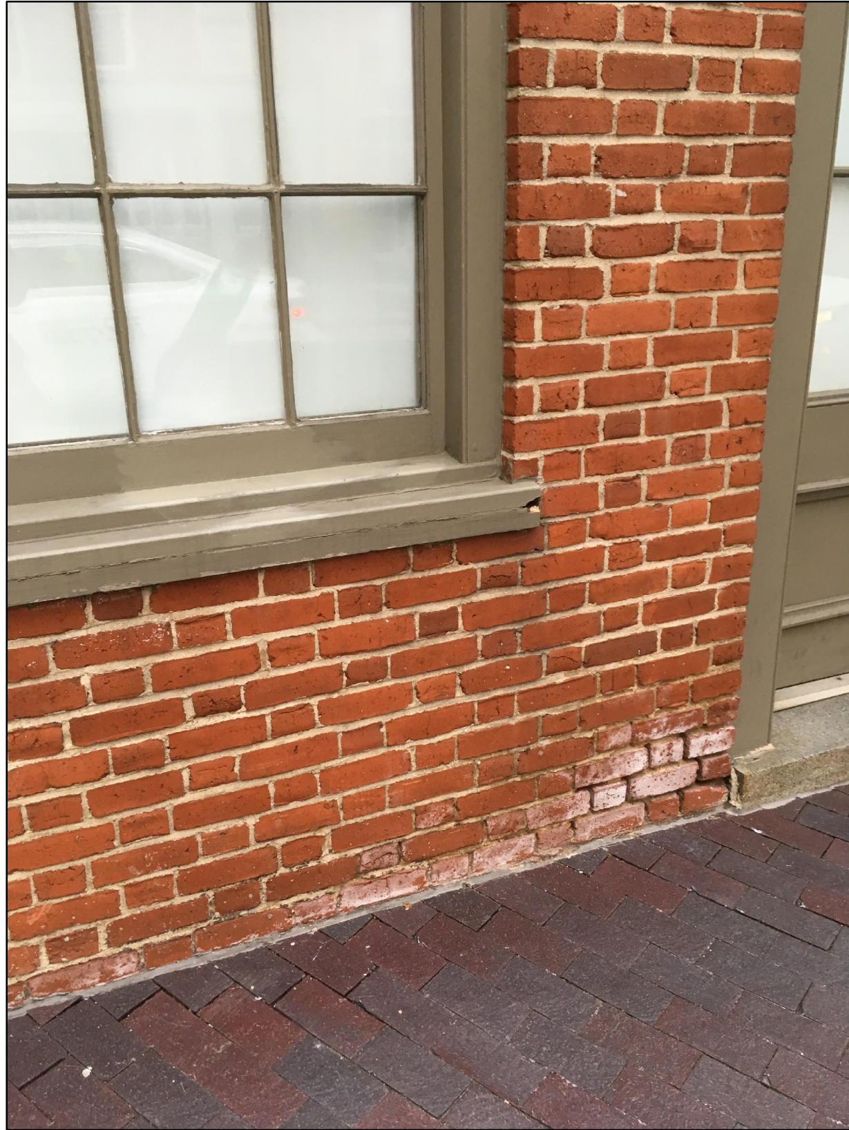
1 EXTERIOR WALL- BRICK & MORTAR DAMAGE
