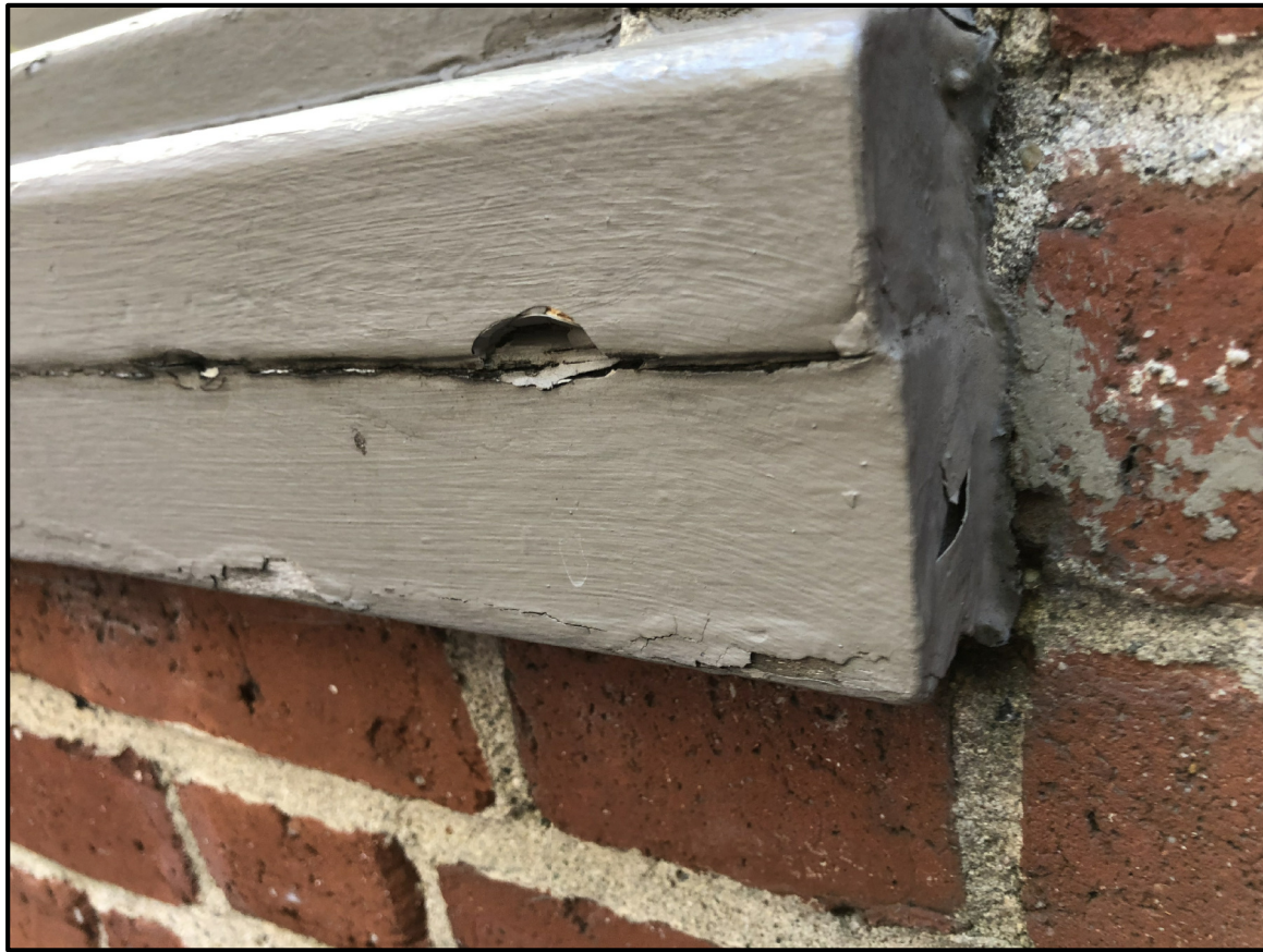
1 WINDOW SILL DAMAGE
