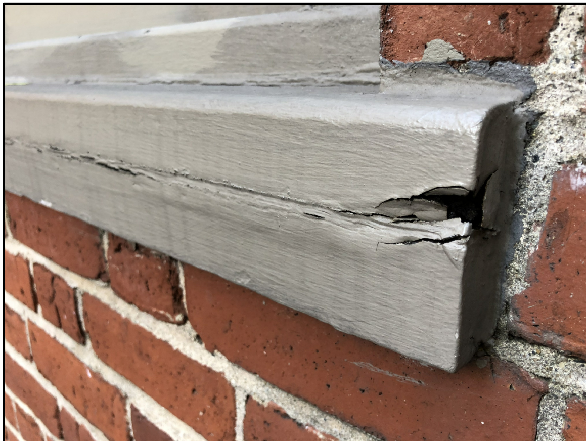
3 WINDOW SILL DAMAGE
