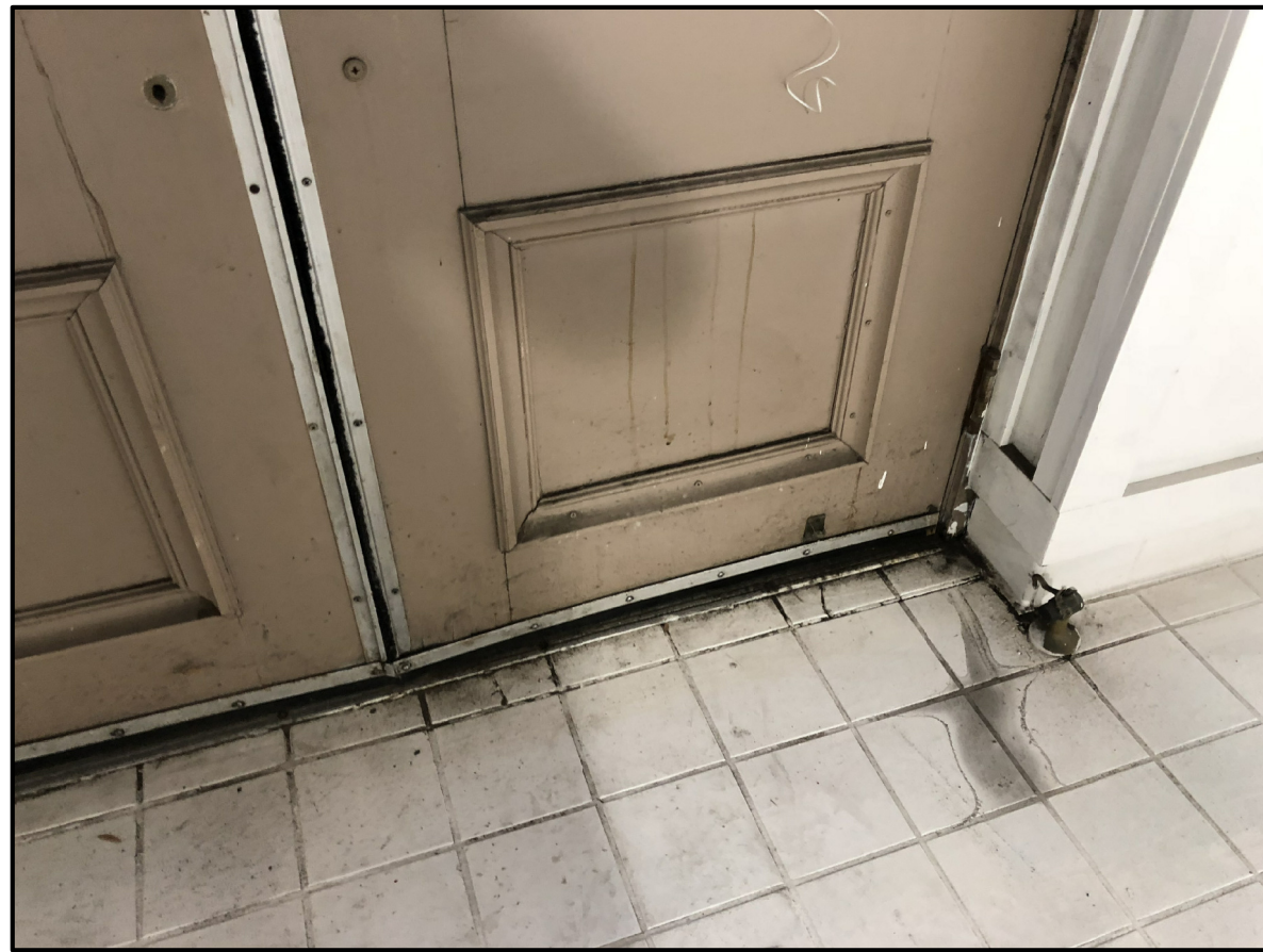
1 DOOR DAMAGE @ INTERIOR
