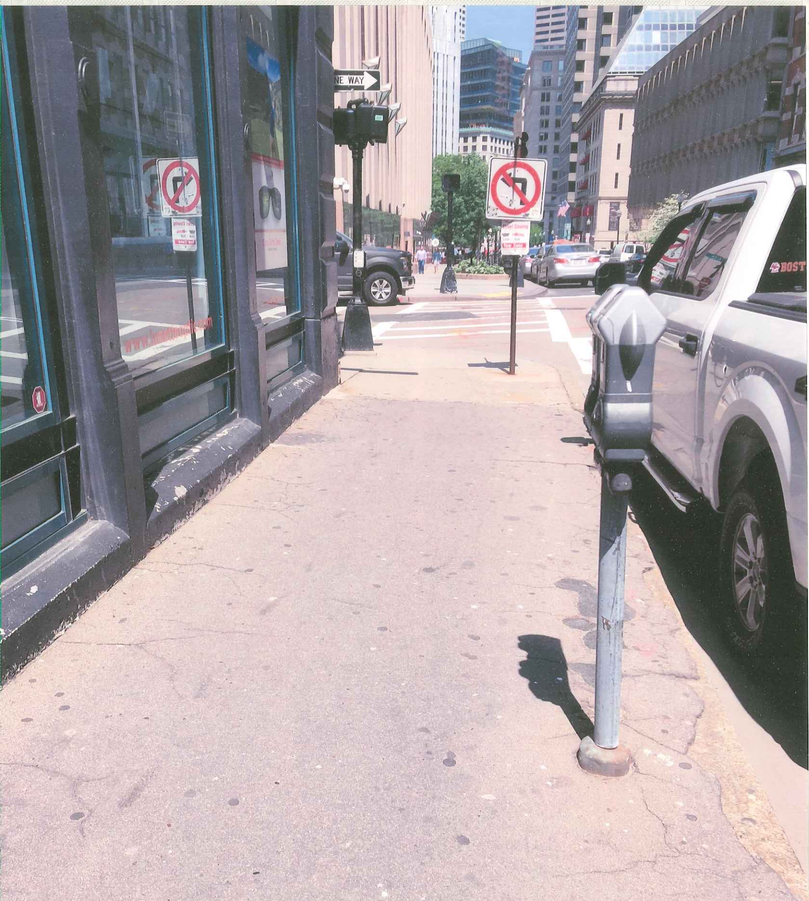
Pearl Street Sidewalk with Vault Below
