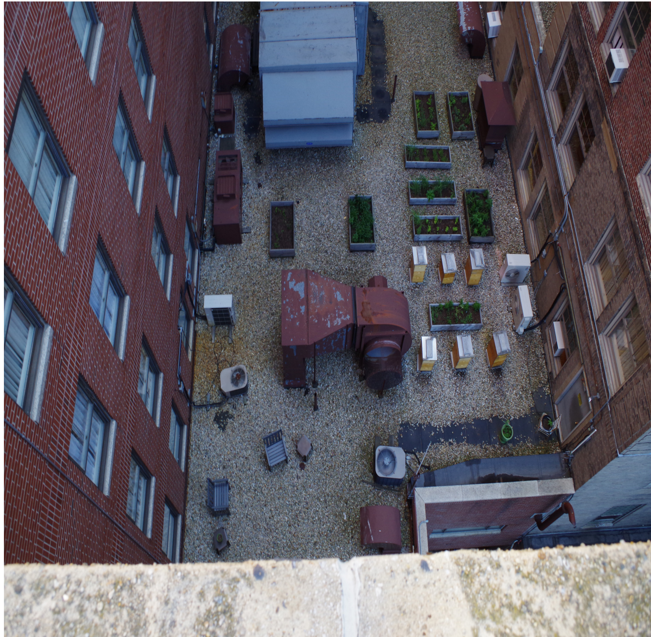
HVAC EQUIPMENT AT ADJACENT BUILDING
