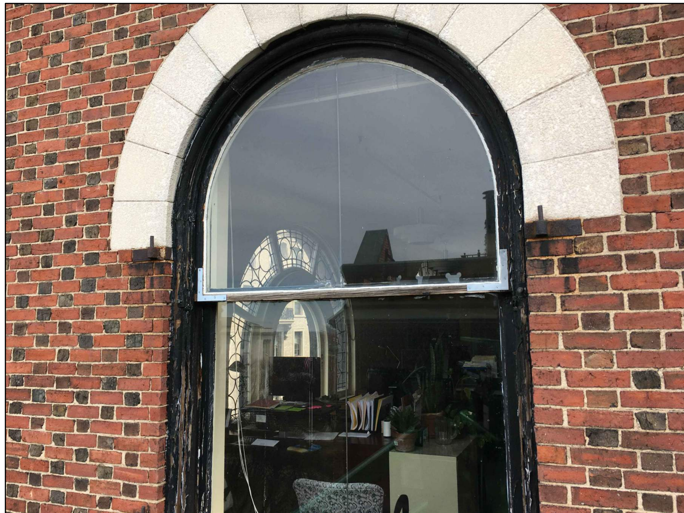
DETERIORATED BRICK MOULD AND SASH
