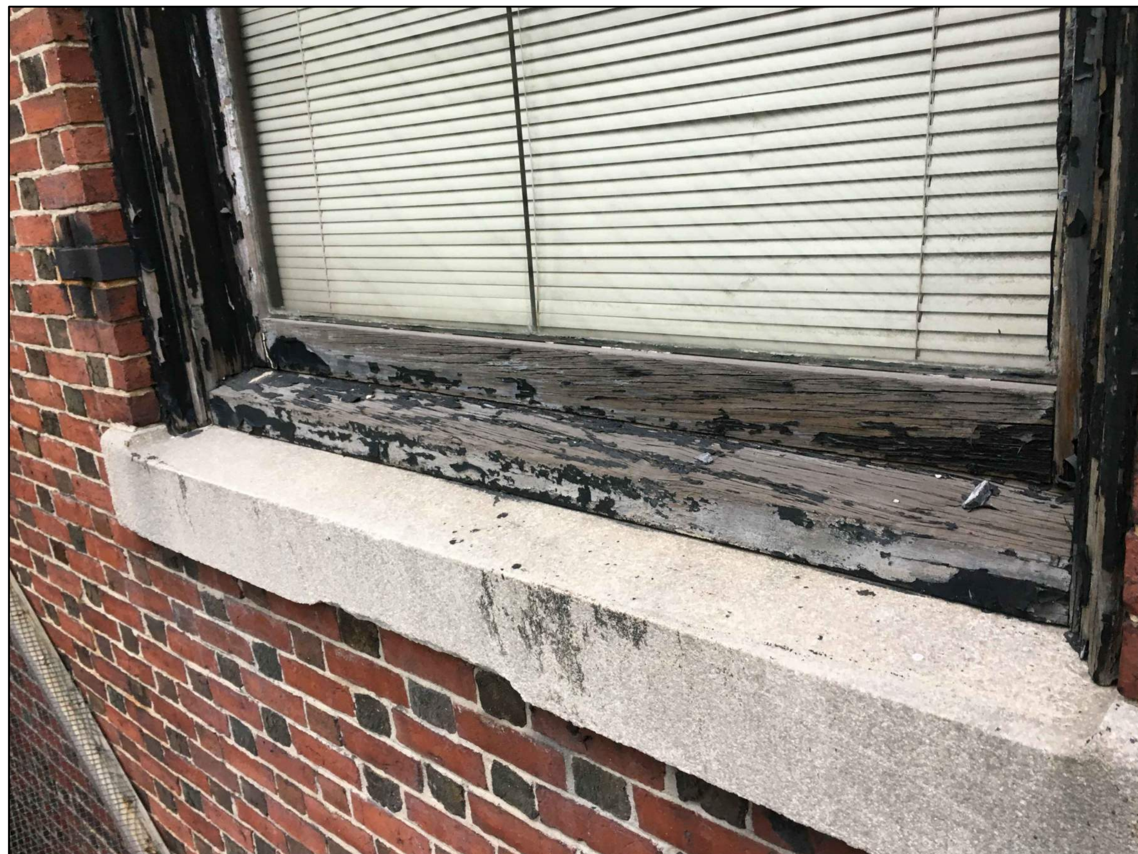
DETERIORATED WOOD SILL AND BRICK MOULD
