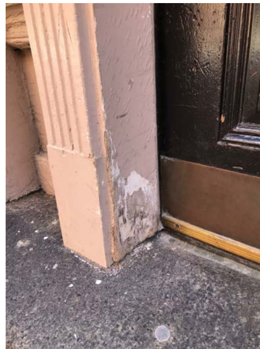
AREAS OF DETERIORATION TO BE REPAIRED
