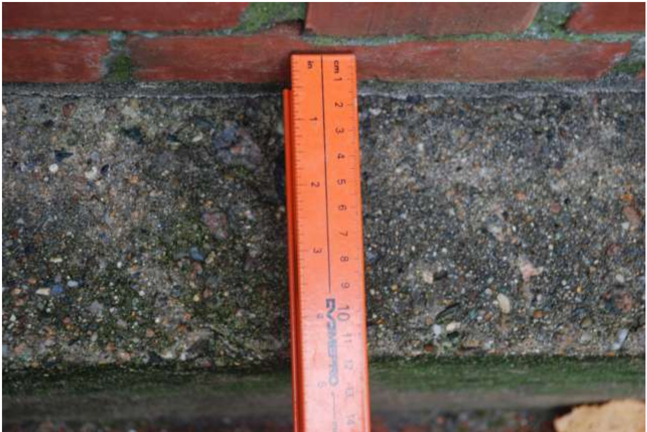
This photo was taken standing in the 183 Comm Ave parking area to measure the setback of the brick wall from the foundation curb.
