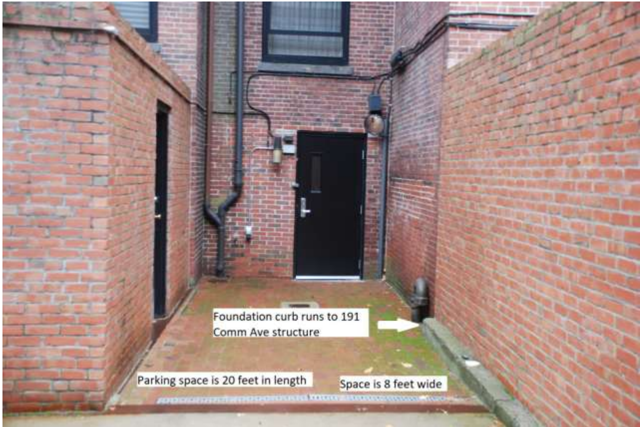
This photograph is taken while standing in Public Alley 425 looking at the rear of 183 Comm Ave.
