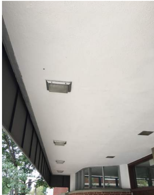
Berkeley Street Entry Canopy Lighting
