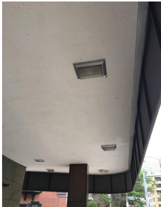
Berkeley Street Entry Canopy Lighting
