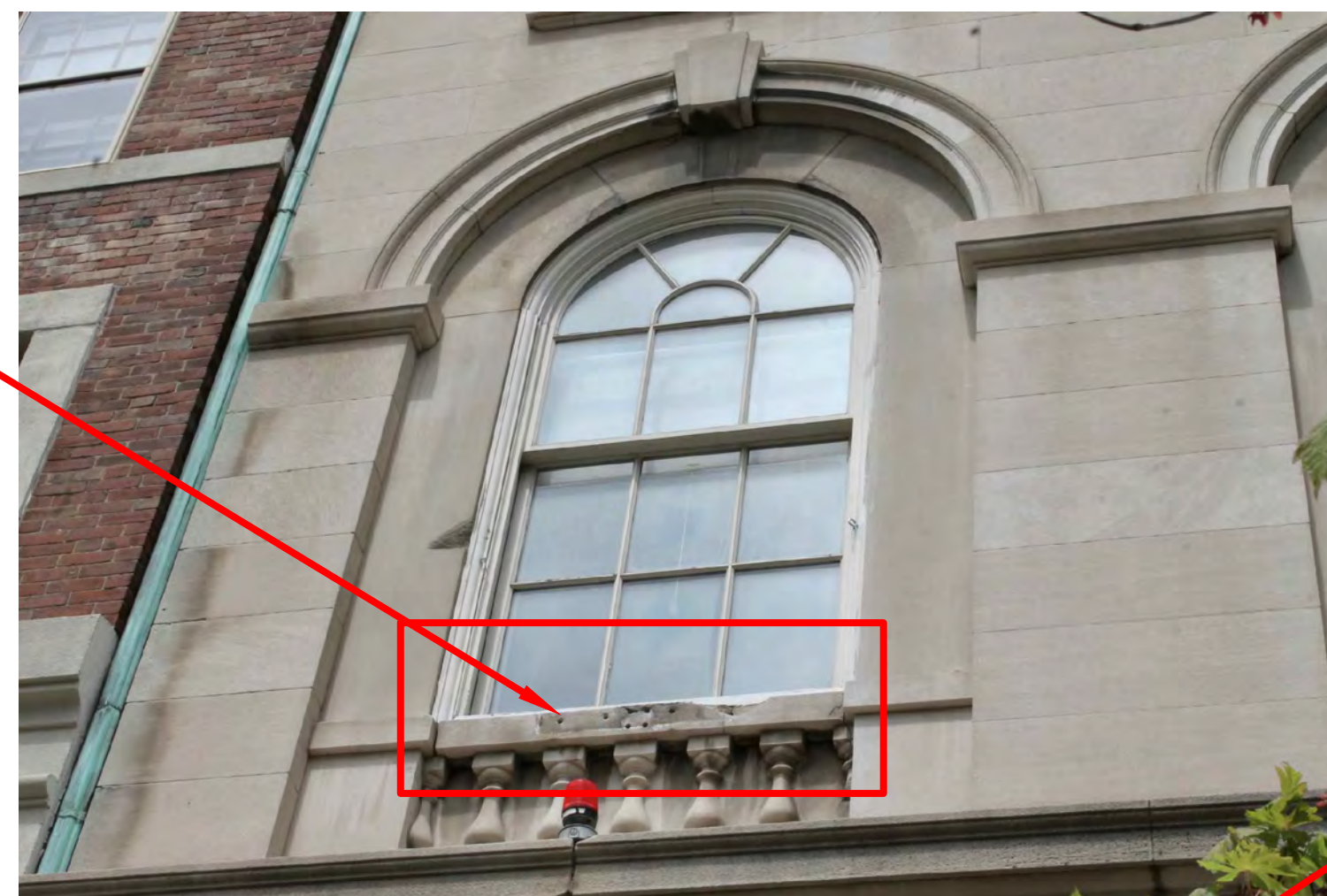
DAMAGED LIMESTONE SILL
