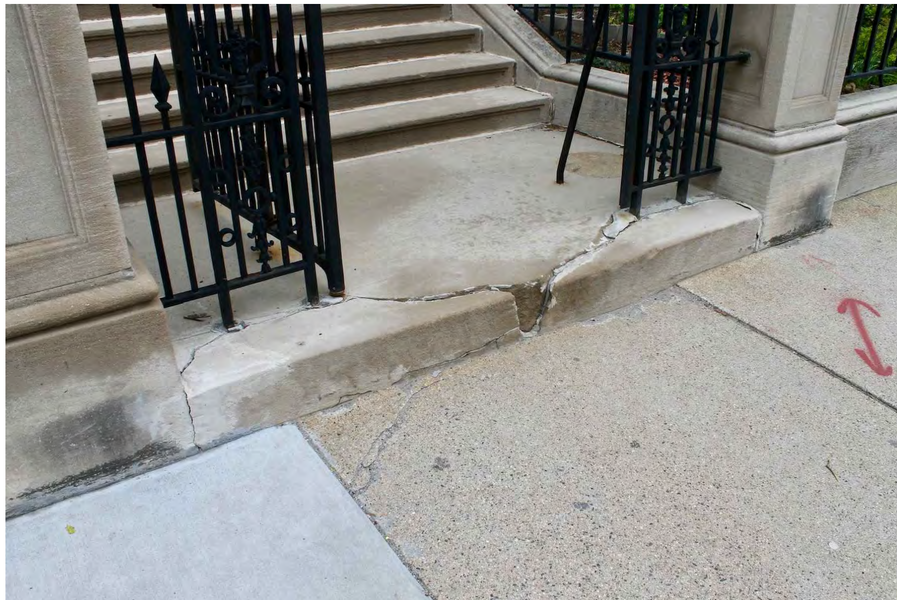
DAMAGED LIMESTONE STEP WITH IRON GATE
