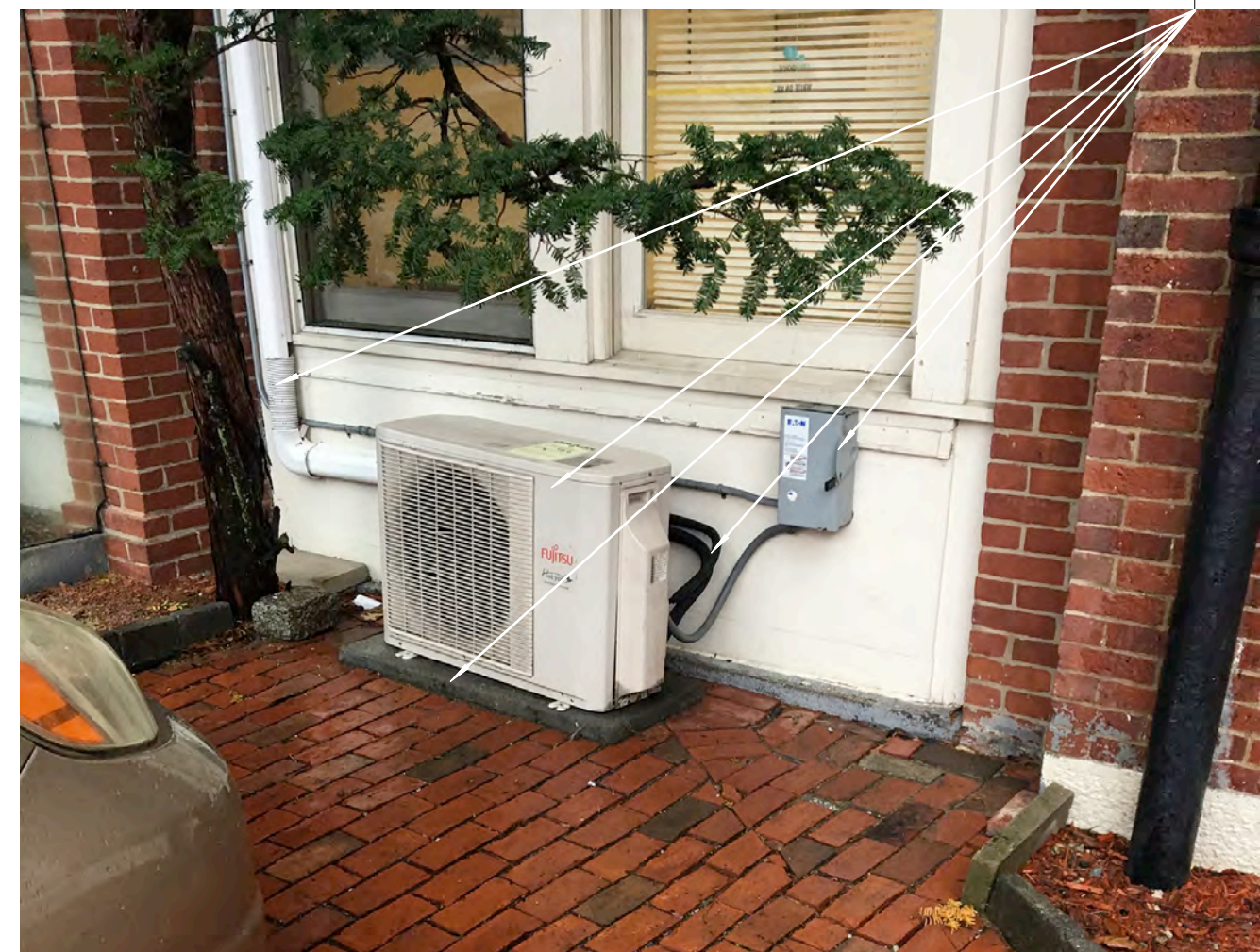
3 PHOTO - EXISTING CONDENSER UNIT AT YARD SCALE: N/A
