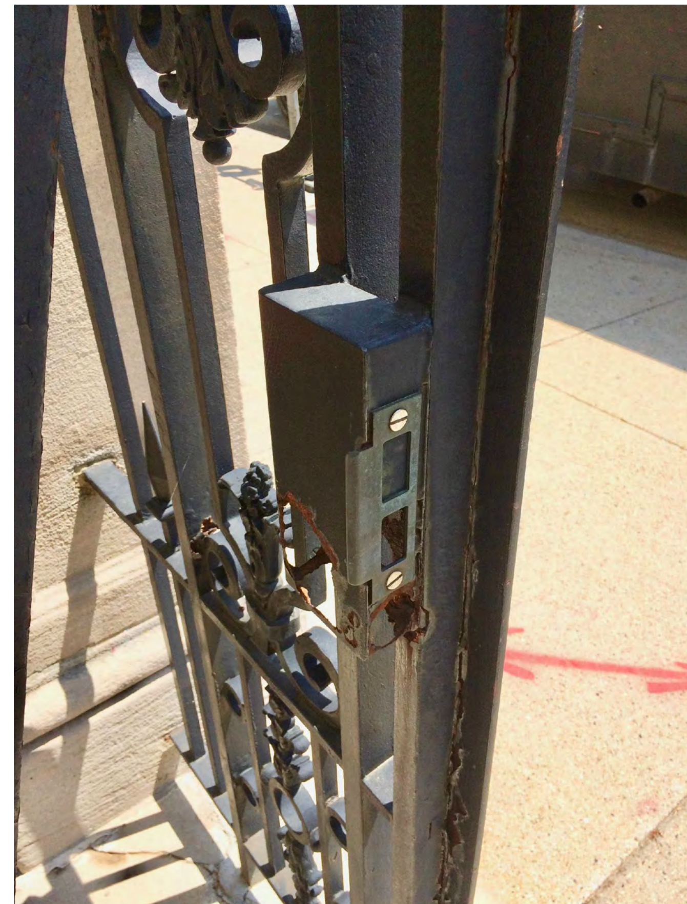
DAMAGED FRONT GATE LATCH
