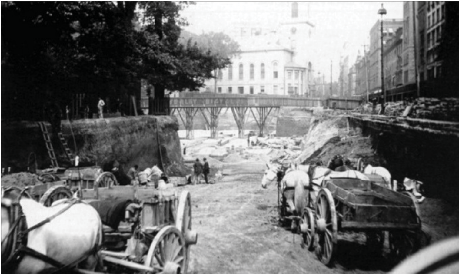
1897 circa – Construction of subway tunnel (current MBTA Green Line) taken near present day Parkman Plaza. Courtesy Boston Public Library
