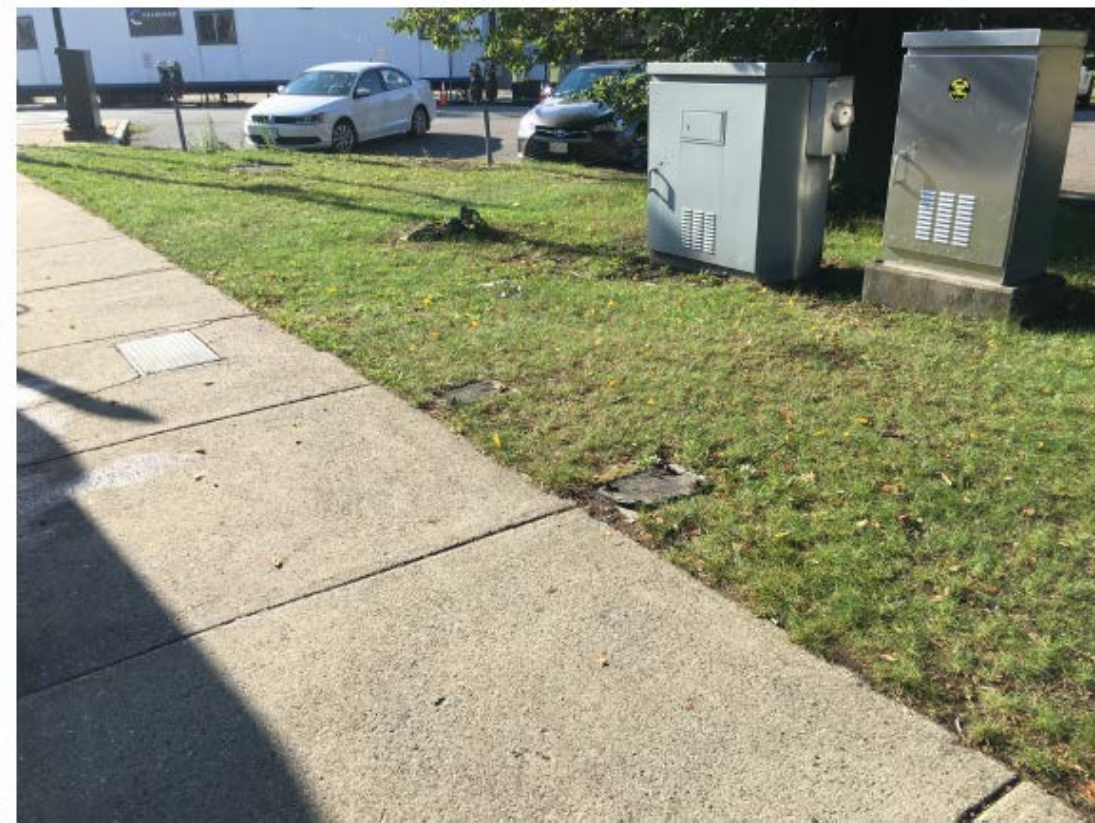
Figure 6 - Control Cabinet (left) to be Replaced in Kind on Existing Foundation, Battery Backup (right) to be Retained
